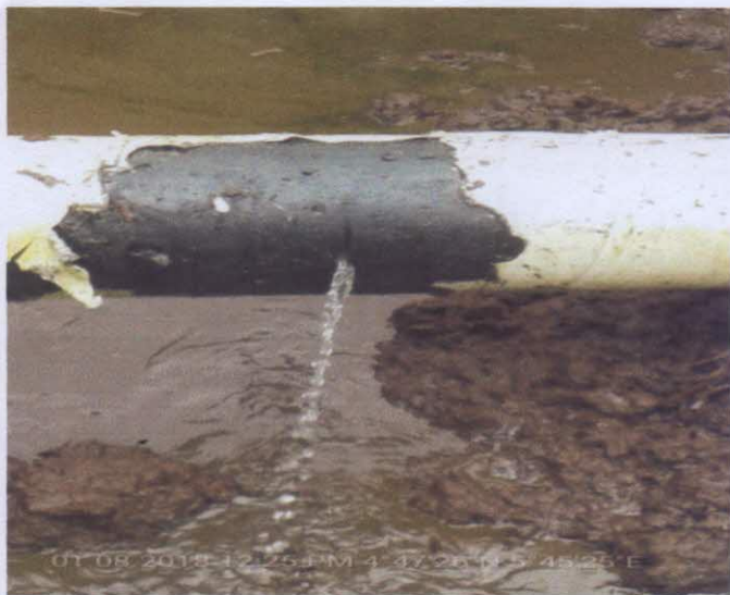
Figure 1: Hacksaw cut on the Pipeline.
