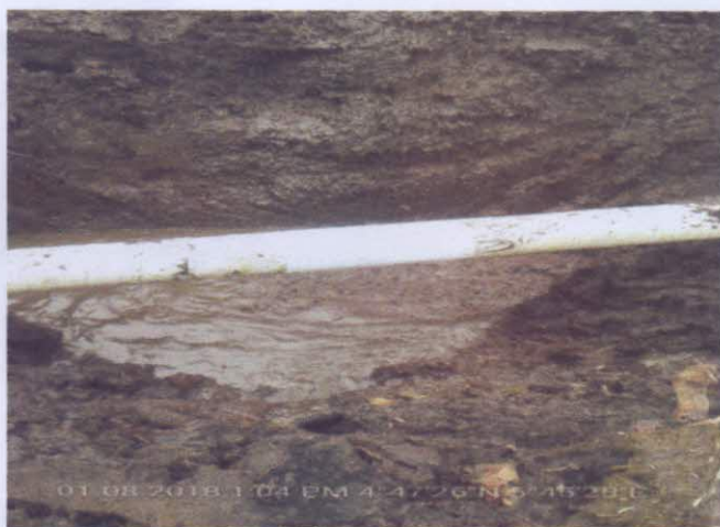
Figure 4: Wrapped section on the Pipeline.
